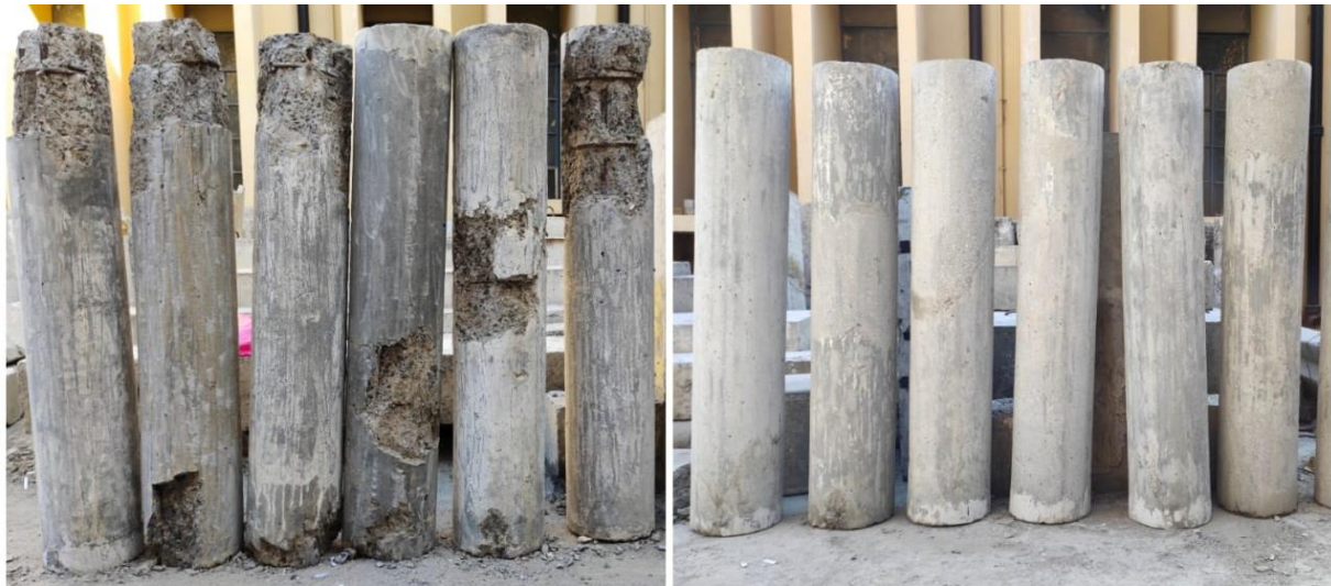
Figure 1.: Already damaged columns on left, on right epoxy and mortar repaired columns
