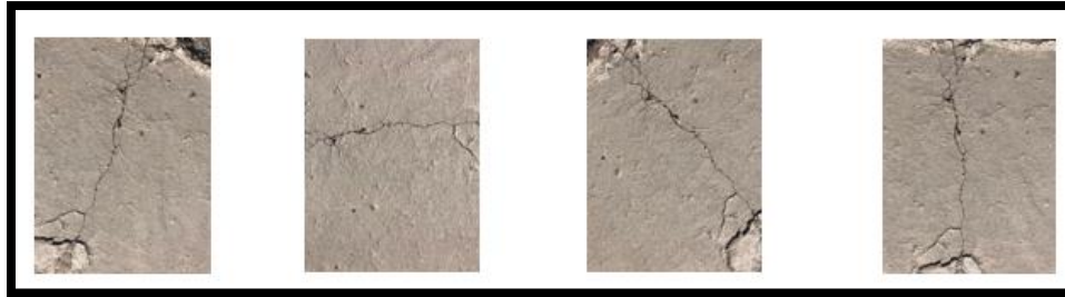
Figure 3: Pavement Cracks of UET Taxila
