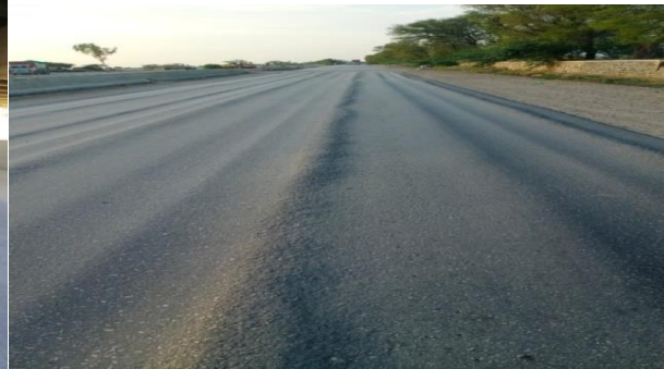
Fig: 3 Severe Rutting after Bridge due to elevated pavement temperature (N-55)
